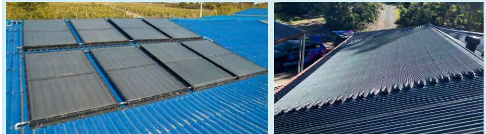
Pool Heating Collectors
