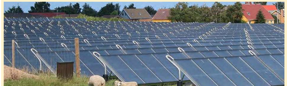
Solar District Heating Plant
