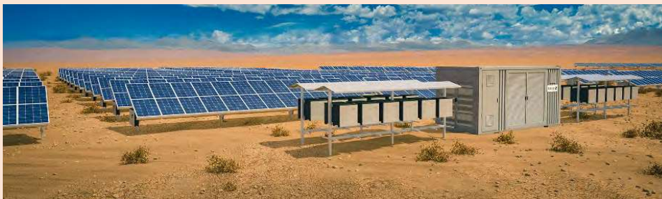
A solar PV farm connected to the grid
