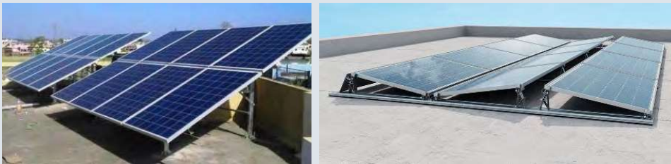
Roof Mounted PV Installations
