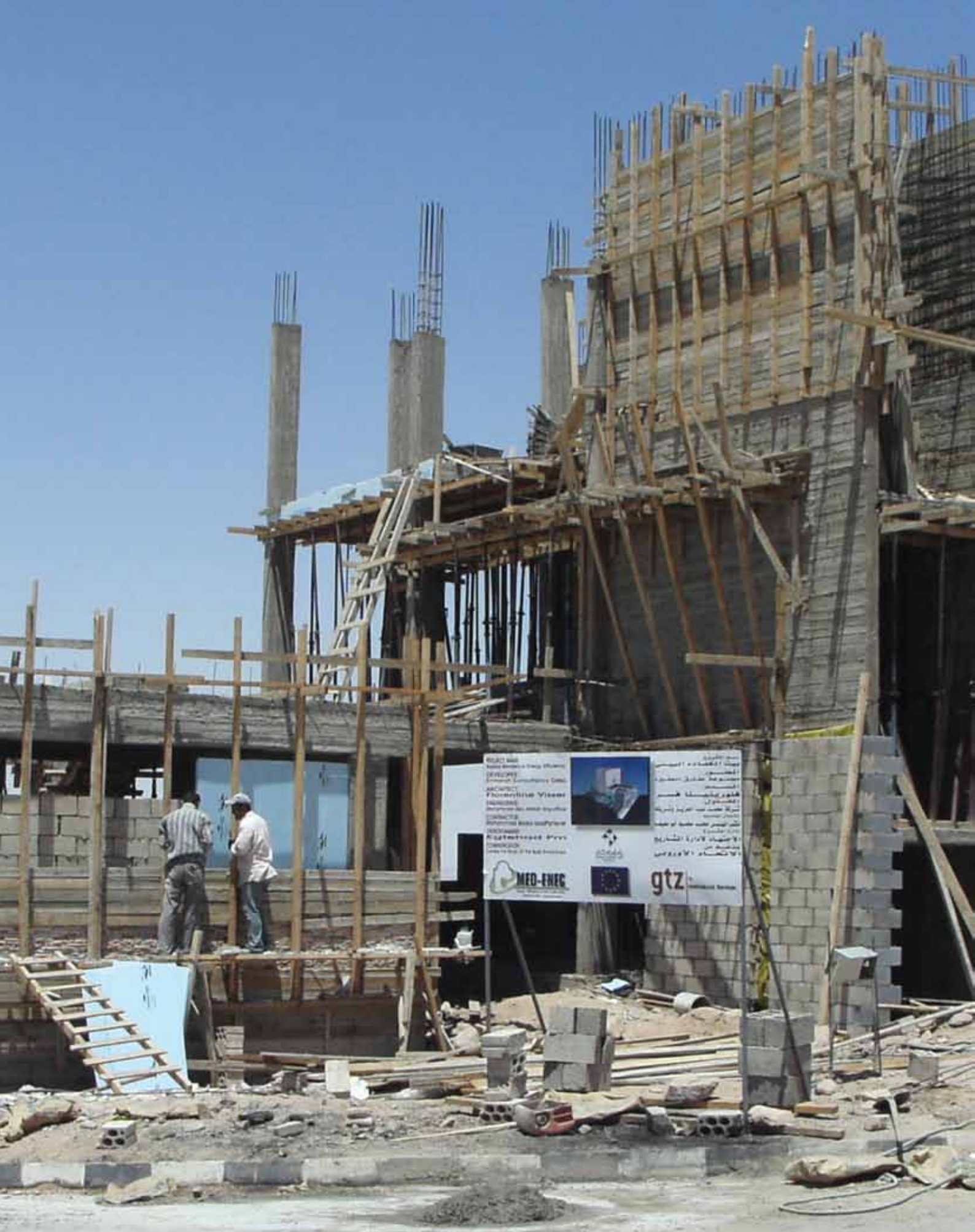
The Aqaba Residence Energy Efficiency project (AREE), Jordan, under construction, was designed according to the passive design approach. The EE measures generated 32% savings on the net energy demand and added 12% to the construction costs, compared to conventional buildings. However, it was calculated that these additional cost would be recovered by a lower energy bill in less than four years. Architect: Florentine Visser
