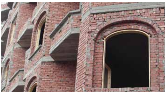
Thermal bridges are very common in the MENA region
