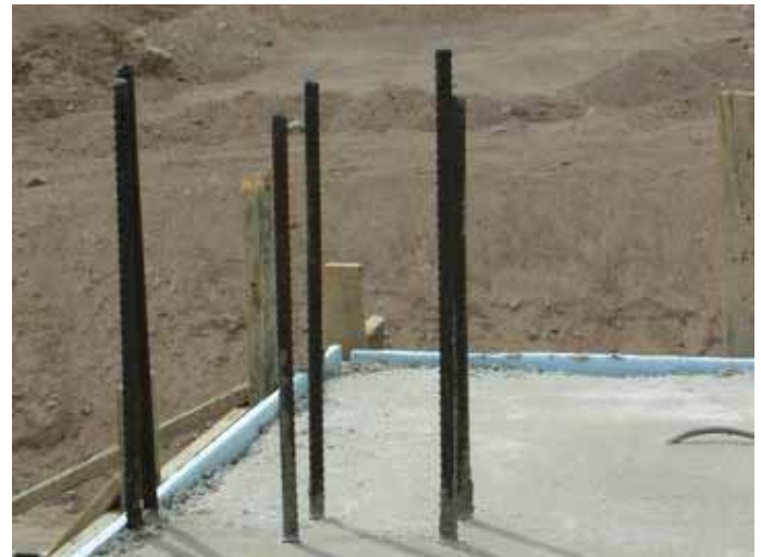
Solving a thermal bridge: 3 cm polystyrene in the formwork before pouring concrete
