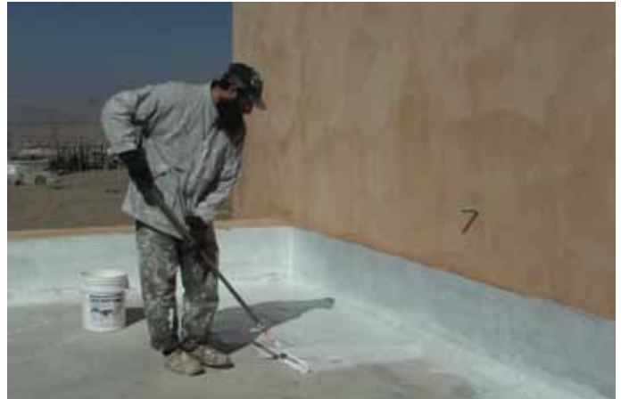
A white roof reduces the cooling load
